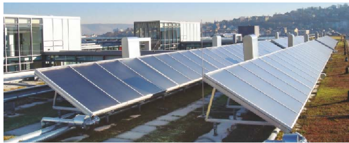
Fig. C2.27 Glass-covered flat collectors and foil collectors for heating of drinking water
