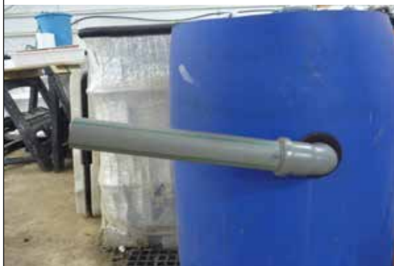
FIGURE 9.13 Overflow pipe on a biofilter
