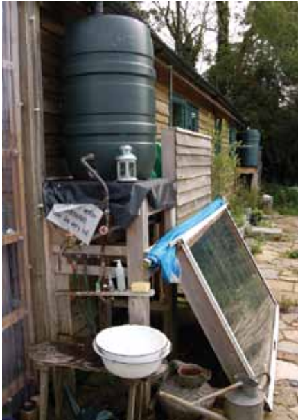
An excellent solar hot water system at Ourganics making full use of both gravity and the thermosyphon effect
