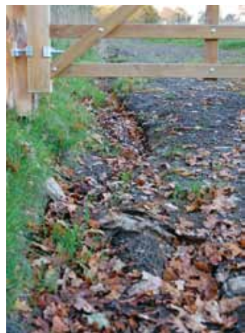
Water run off erosion gully
